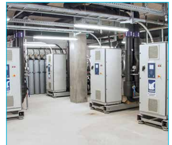
Complete chiller plant
